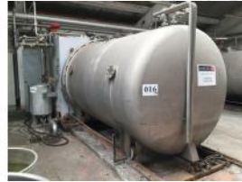
Reference: SAS-016 Jigger high temperature Year: 1984 Brand: MCS Width: 2600
