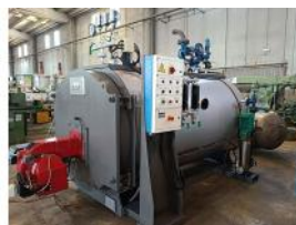
Reference: AV7-014 STEAM BOILER 1750kg Year: 2016 Brand: PERELLÓ I.VAR Width: .
